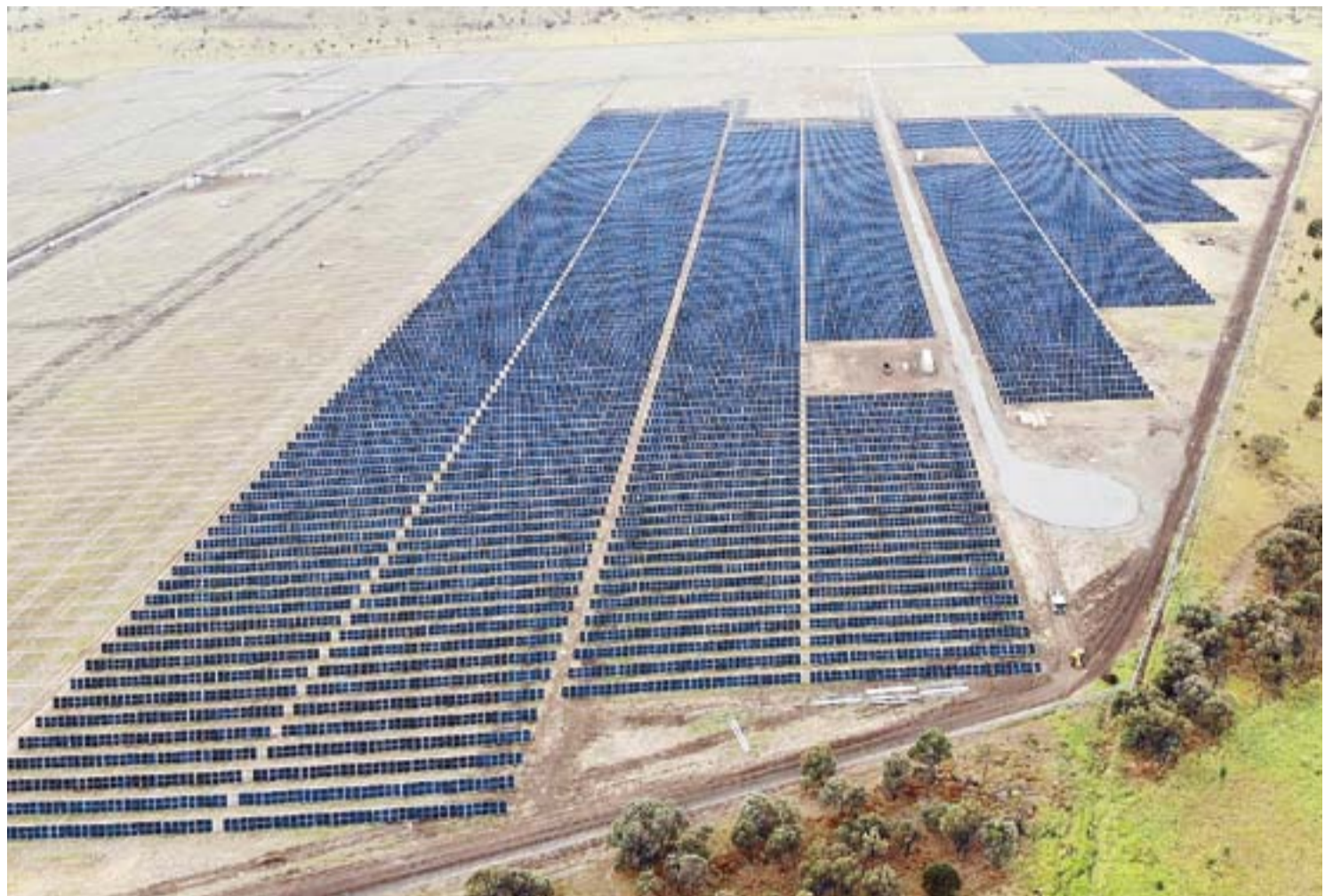
CS Energy has added more than 300 megawatts of contracted renewables to its portfolio in recent years including the Moura Solar Farm. Picture: SUPPLIED
