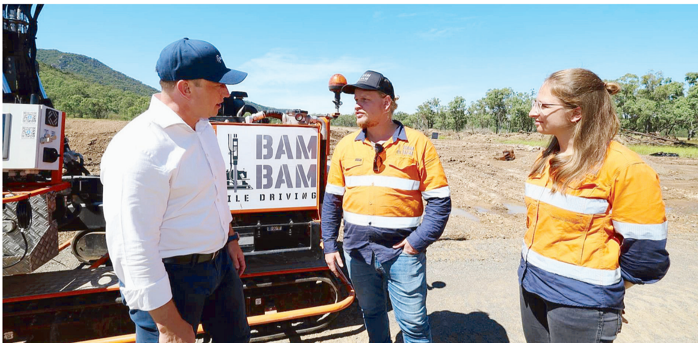
Premier Steven Miles met with local tradespeople earlier this month who have begun the construction of Aldoga Solar Farm. Pictures: SUPPLIED
