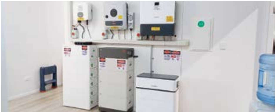
The innovative battery system and inverter display.
